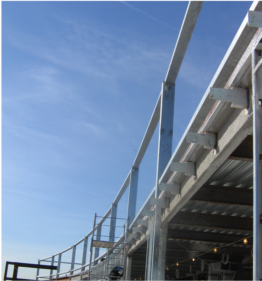
Installed Steel Mounting Tabs at Coppin State University Health and Human Services Building
